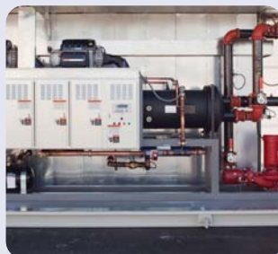
Chillers and Chiller Plants
